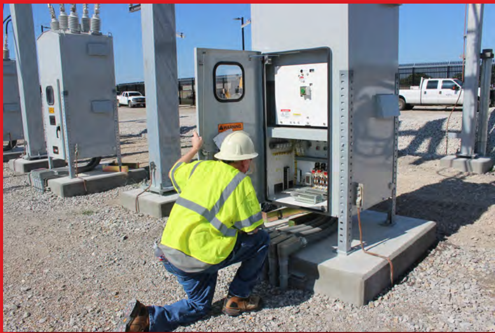
Inspecting equipment in the rebuilt Apollo Substation, 2020. Garland Power & Light Collection
