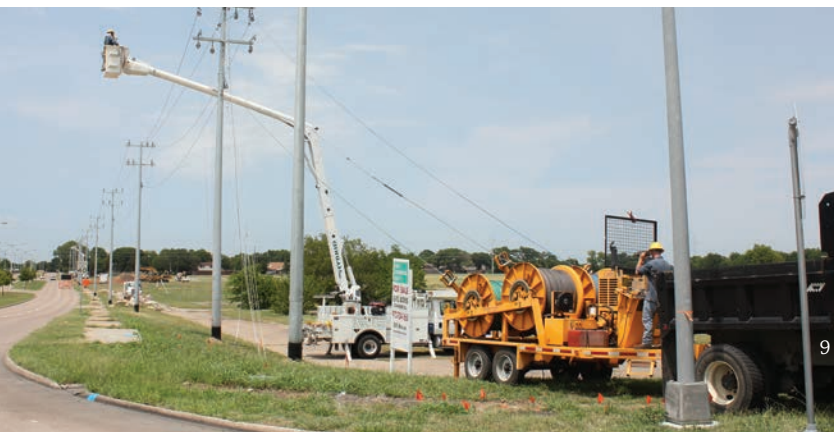
New Rosehill distribution feeder
