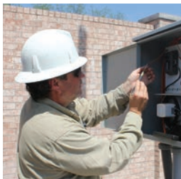
Substation security equipment
