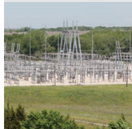
TMPA transmission facility
